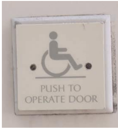
Figure 4: Automatic door opener, with large push button.
