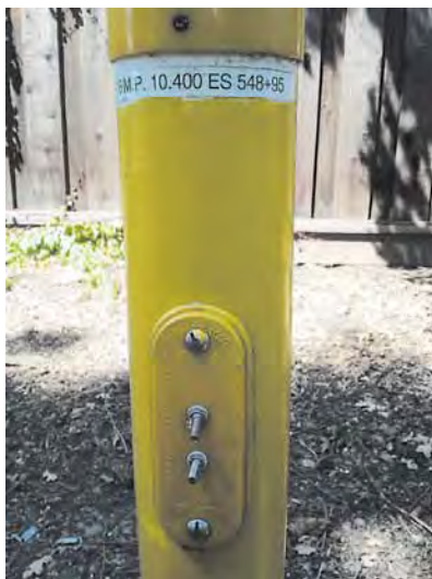
Cathodic protection test point along the Iron Horse Corridor
