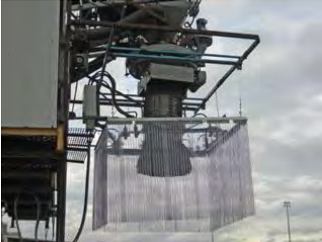
Figure II-3: Wind Barrier surrounding a transfer point
