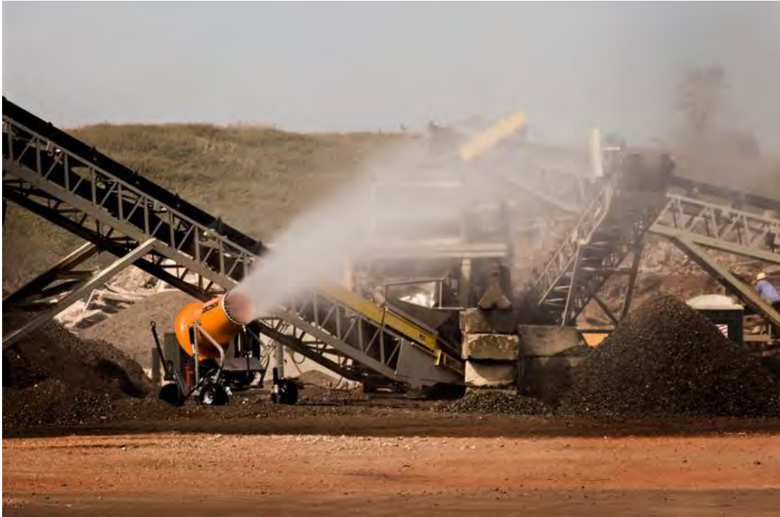
Figure II-4: Use water fog or mist to control dust during active handling operations.
