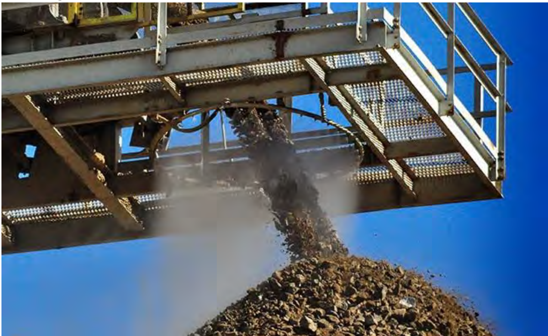
Figure II-5: Spray water fog and mist to keep disturbed surfaces damp during bulk material moving operations.
