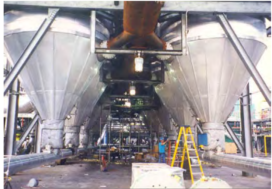
Aeropulse Carbon Black Factory
