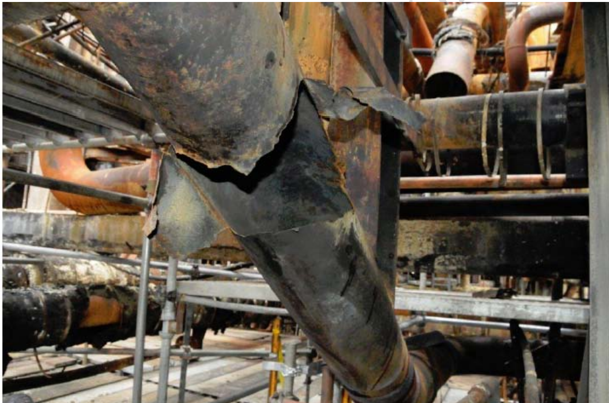
Figure 7. Photo of rupture on 4-sidecut 52-inch component
