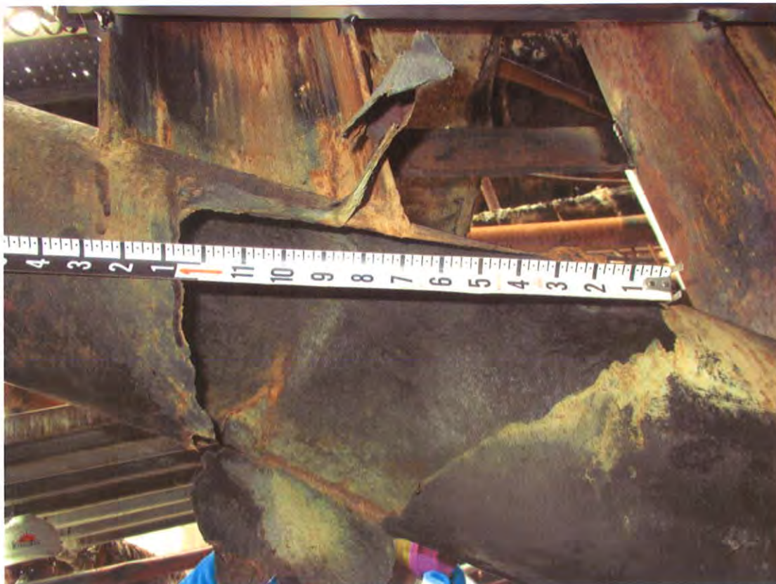
Figure 8. Close-up photograph of the ruptured pipe component taken during the inspection prior to removal.
