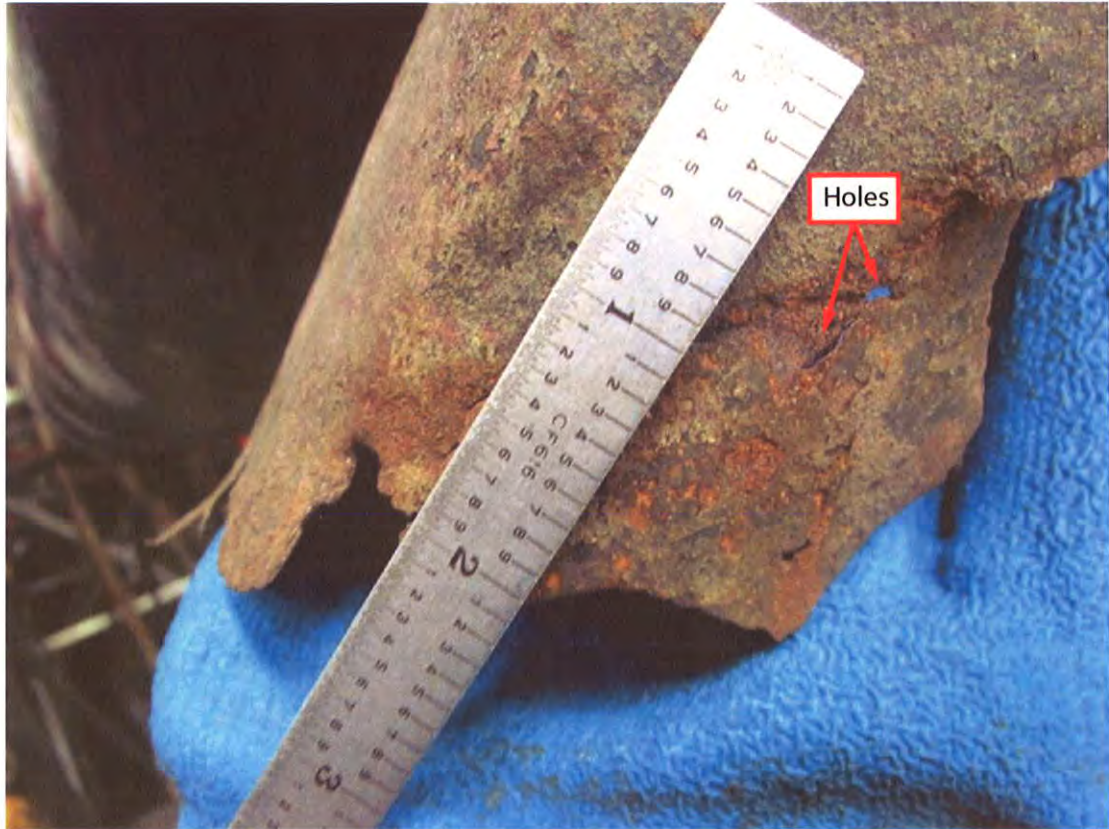
Figure 10. Photograph of one of the metal flaps associated with the 4SC rupture. Small perforations are visible in the flap.
