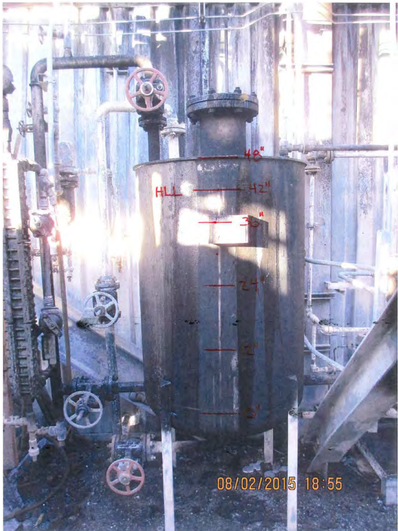
PICTURE OF DAY TANK WITH LEVELS MARKED
