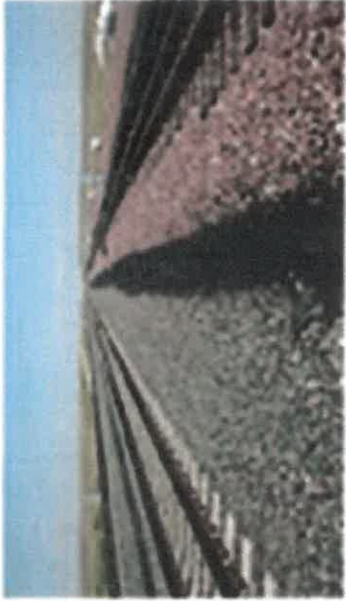
Note coal dust deposit in ballast drainage area
