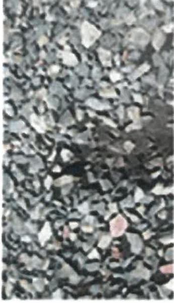
What is below ballast when you "scratch the surface"
