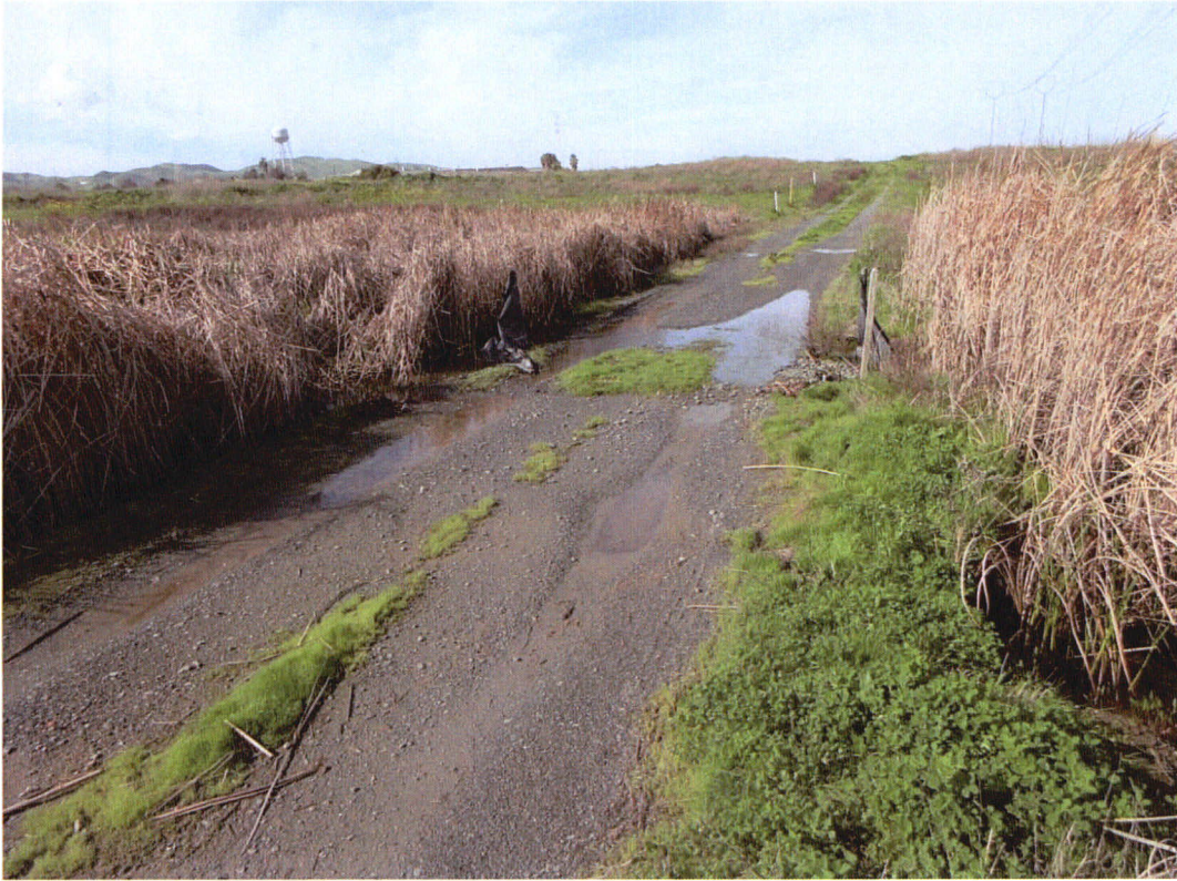
Photograph 7. Gravel Road near the Outfall (Location A). February 21, 2017.
