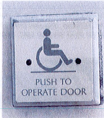
Figure 4: Automatic door opener, with large push button.
